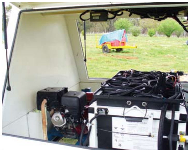
◀ Figure 1b: The Genset, used to keep battery bank voltage above set-point.
