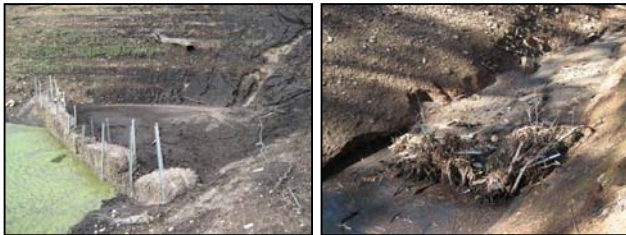
Figure 2 (LH) Algal growth adjoining hay bale sediment trap Figure 3 (RH) Destroyed trap on steep slope
