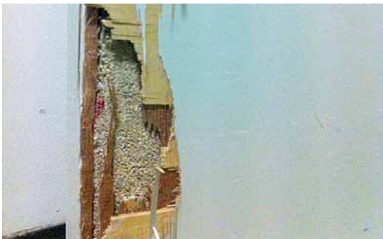
Damaged fire door.
